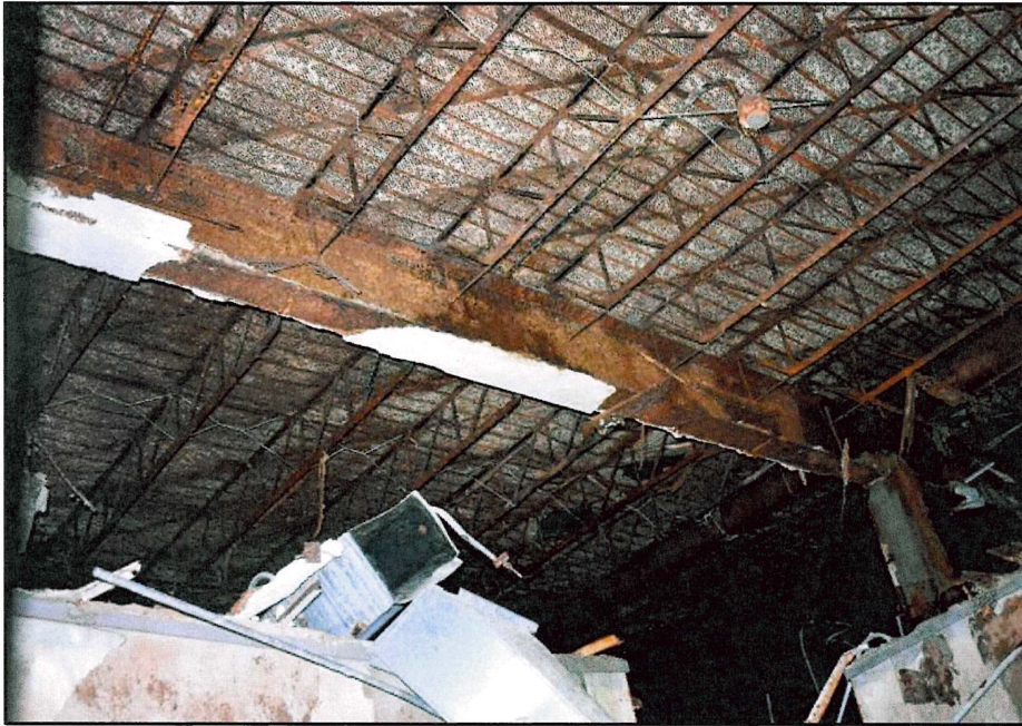
PHOTO NO. 4: Supported floor framing with surface corrosion.
