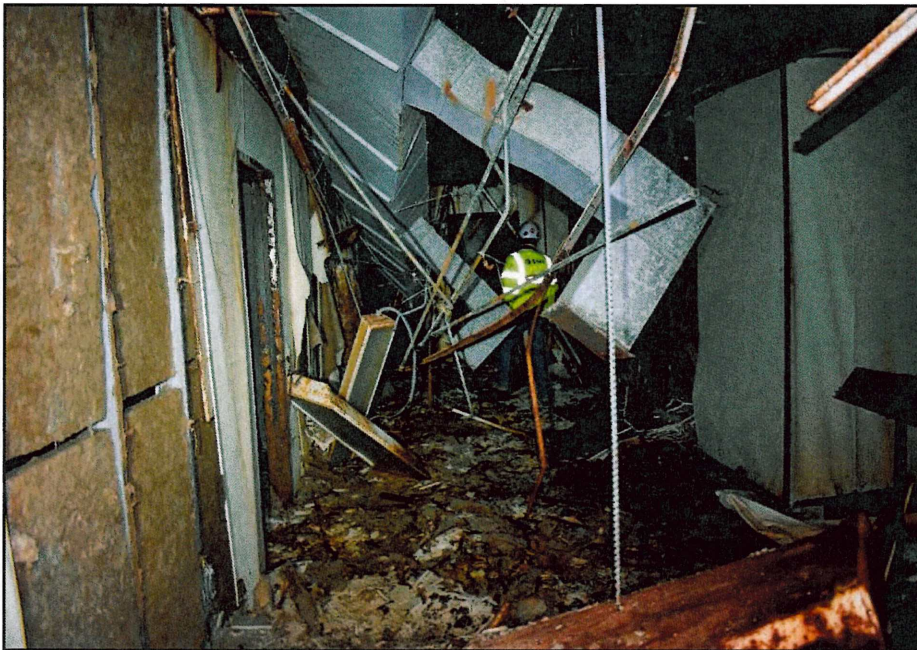
PHOTO NO. 3: Floor area covered with debris; HVAC duct partially hanging from the ceiling.
