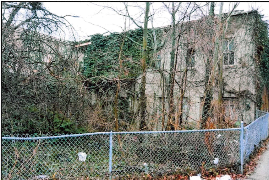
PHOTO NO. 11: Ivy and other growth inhibiting view of north and west exterior walls (building northwest corner) and ravine (between chain-link fence and building) restricted observations of these walls.
