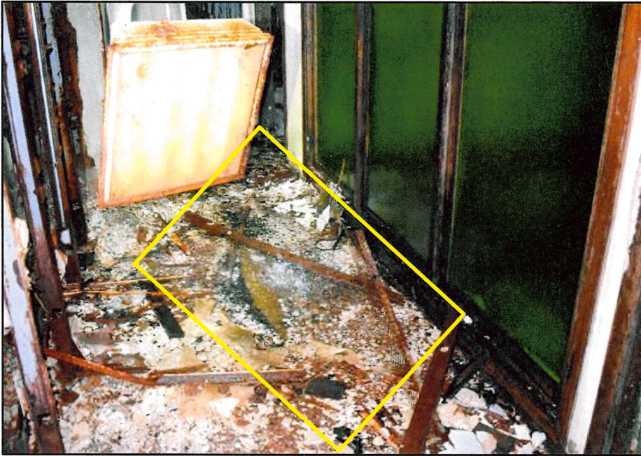
PHOTO NO. 8: Active leak (breach at roof level) and ponding water on second-floor (yellow rectangle).
