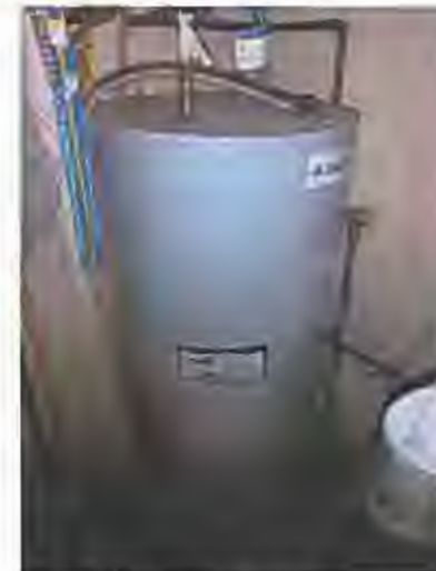
The electric tank serving the leasing office.
