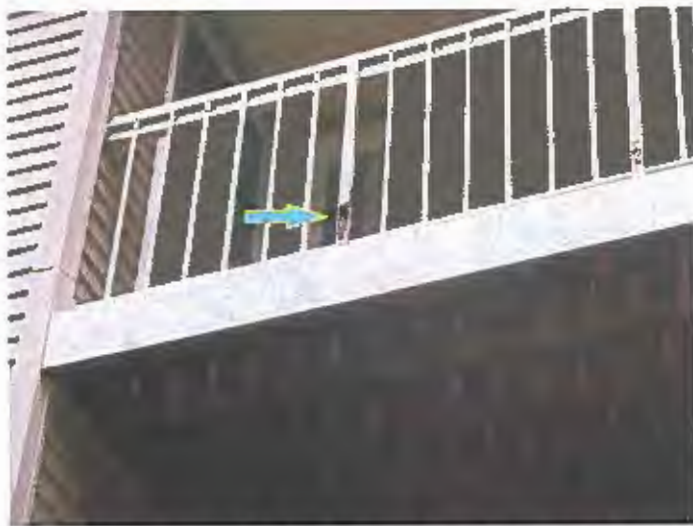
Close up of rust and deterioration of the steel balcony railing post. Arrow pointing to an area that has rusted through.
