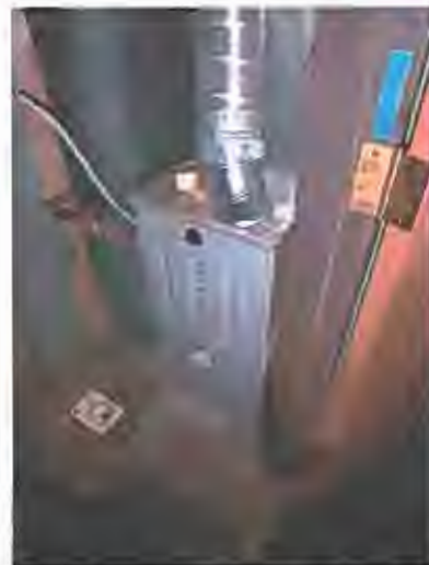
Example of an older Payne gas-fired furnace serving common hallway/stairwells (one of three).
