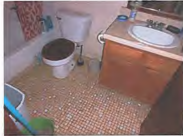
Typical bathroom fixtures and finishes.
