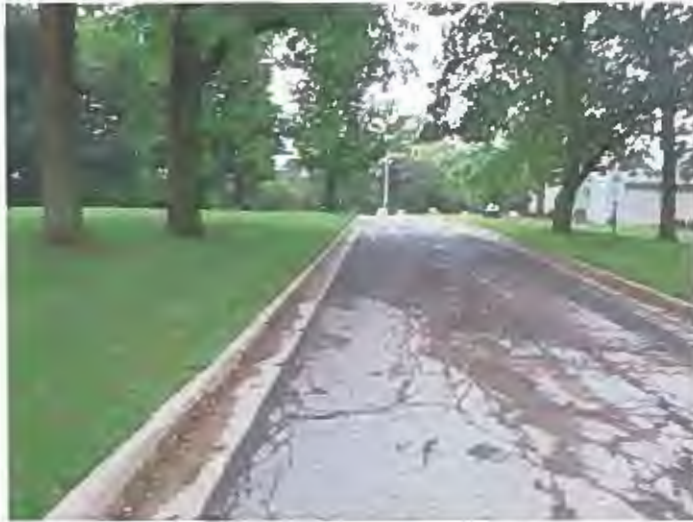
View of the entrance driveway to one of two parking lot areas. The surface exhibits cracking, potholes and age related wear/deterioration.
