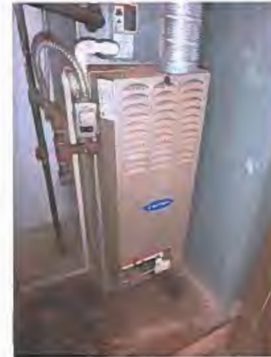
Typical unit level gas-fired warm air furnace located in a mechanical closet on the balcony/patio.
