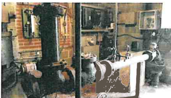
View of interior of pump house.
