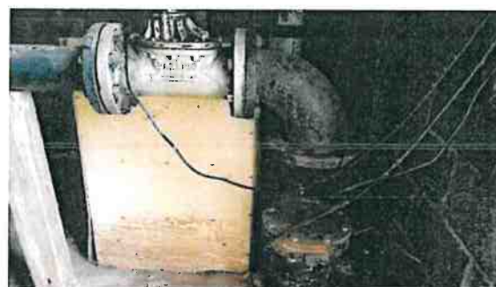
View of interior of pump house, note the pump is not in operation or currently connected.
