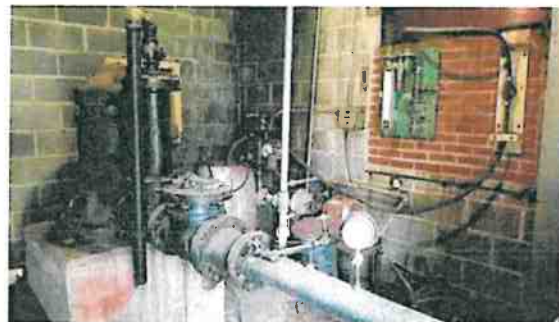
View of interior of pump house.
