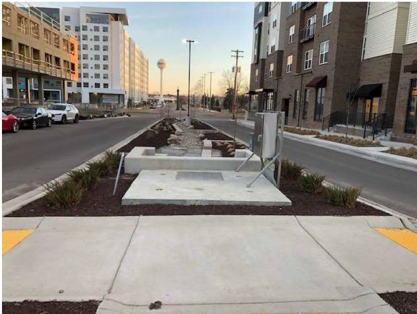
ICDC storm drainage infrastructure located in the median of Cascade Boulevard (looking north toward Michigan Avenue. 3-29-2022
