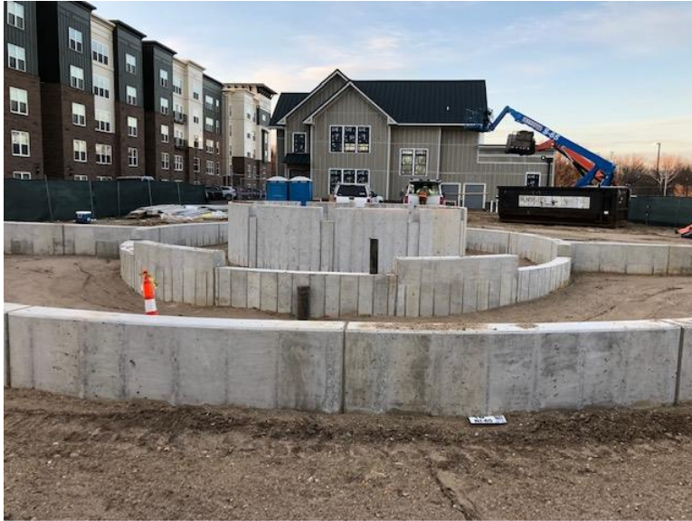
ICDC storm drainage facility and future restaurant located on private property. Looking south in Cascade Boulevard.
