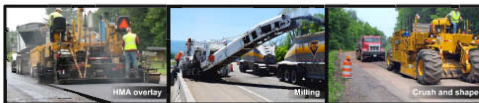
Figure 4 Examples of structural improvement treatments—(from left) HMA overlay on an unmilled pavement, milling asphalt pavement, and pulverization of a road during a crush-and-shape project.
