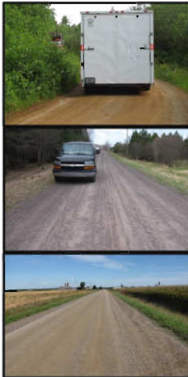
Figure 2: Top – Road with IBR number of 1 road that has poor surface width, poor drainage adequacy, and poor structural adequacy. Middle – Road IBR number of 7 that has fair surface width, fair drainage adequacy, and fair structural adequacy Bottom – Road with IBR number of 9 road that has good surface width, good drainage adequacy, and good structural adequacy
