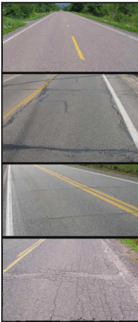
Figure 1 Top image, right – PASER 8 road that is considered “good” by the TAMC exhibit only minor defects. Second image, right – PASER 5 road that is considered “fair” by the TAMC Exhibiting structural soundness but could benefit from CPM Third image, right – PASER 6 road that is considered “fair” by the TAMC. Bottom image, right – PASER 2 road that is considered “poor” by the TAMC exhibiting significant structural distress.
