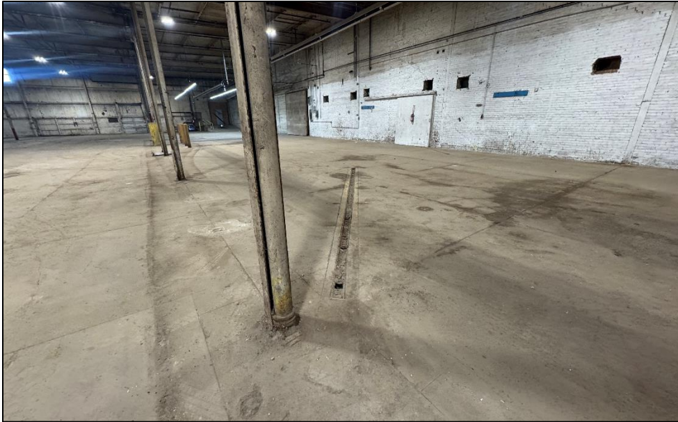
Photo 9: View of trench drain within the subject property building.
