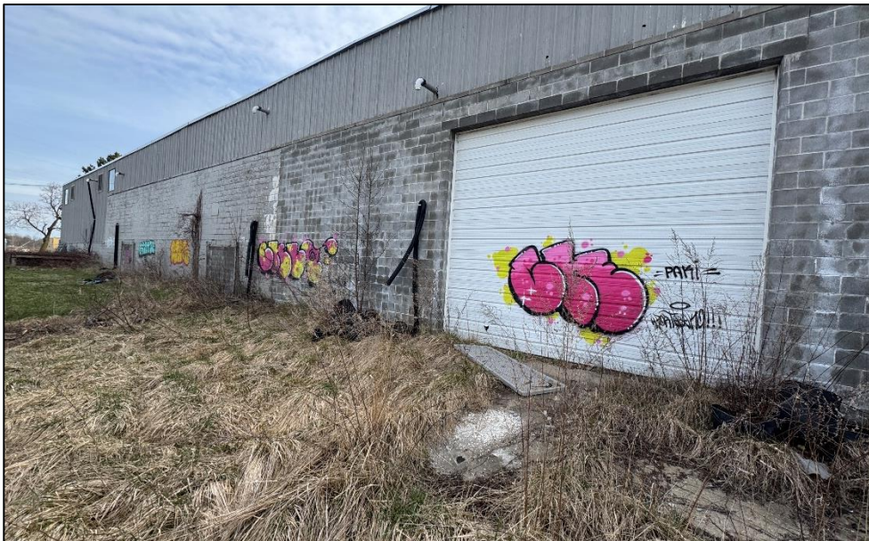
Photo 4: View to the east from the west side of the subject property.
