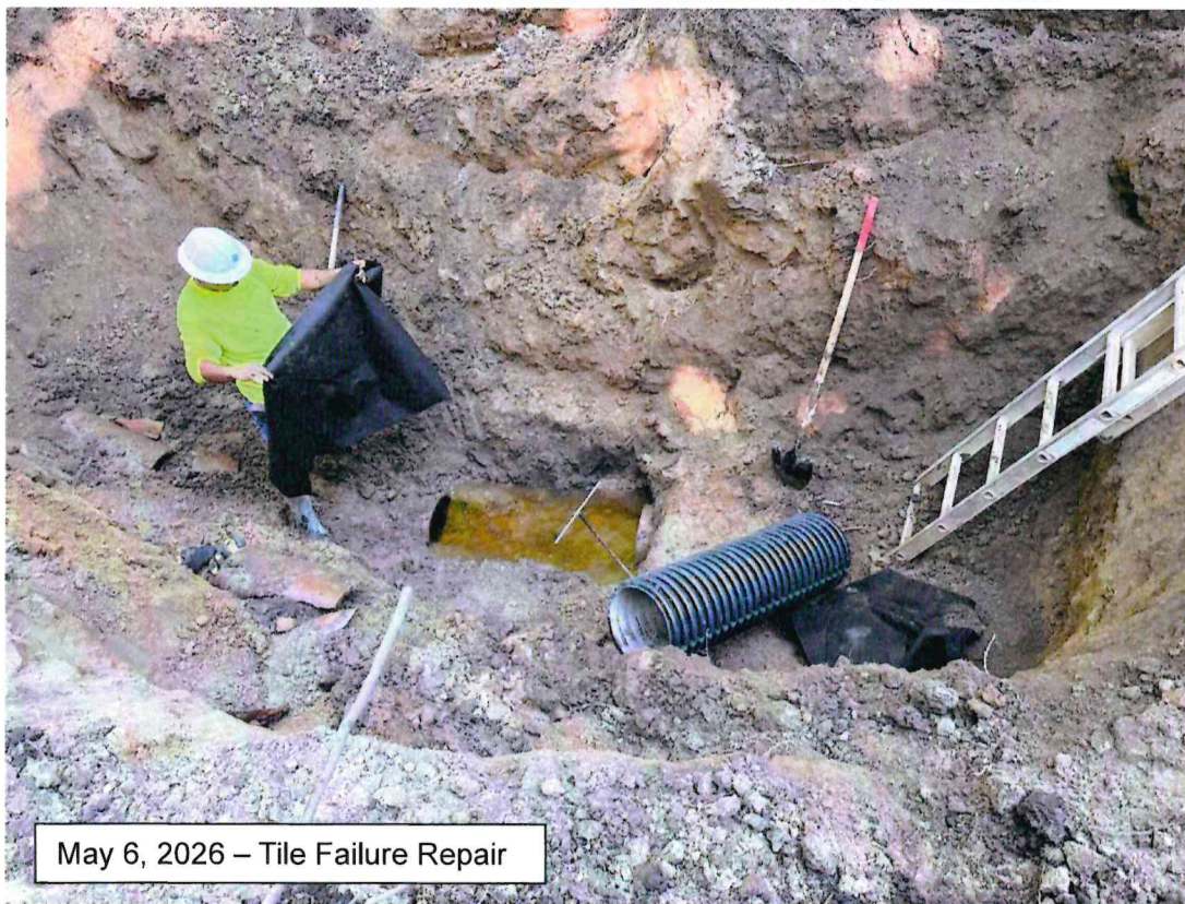
May 6, 2026 – Tile Failure
