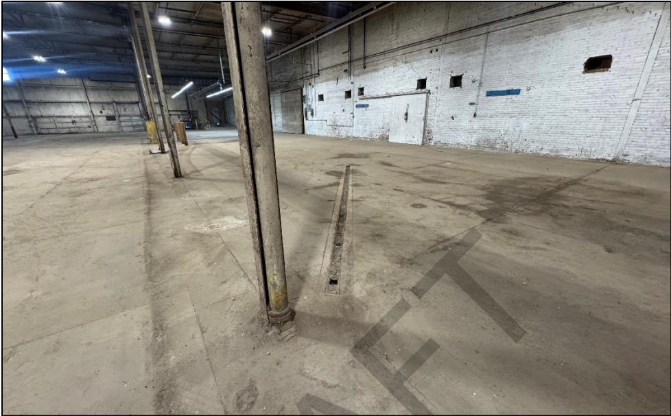
Photo 9: View of trench drain within the subject property building.
