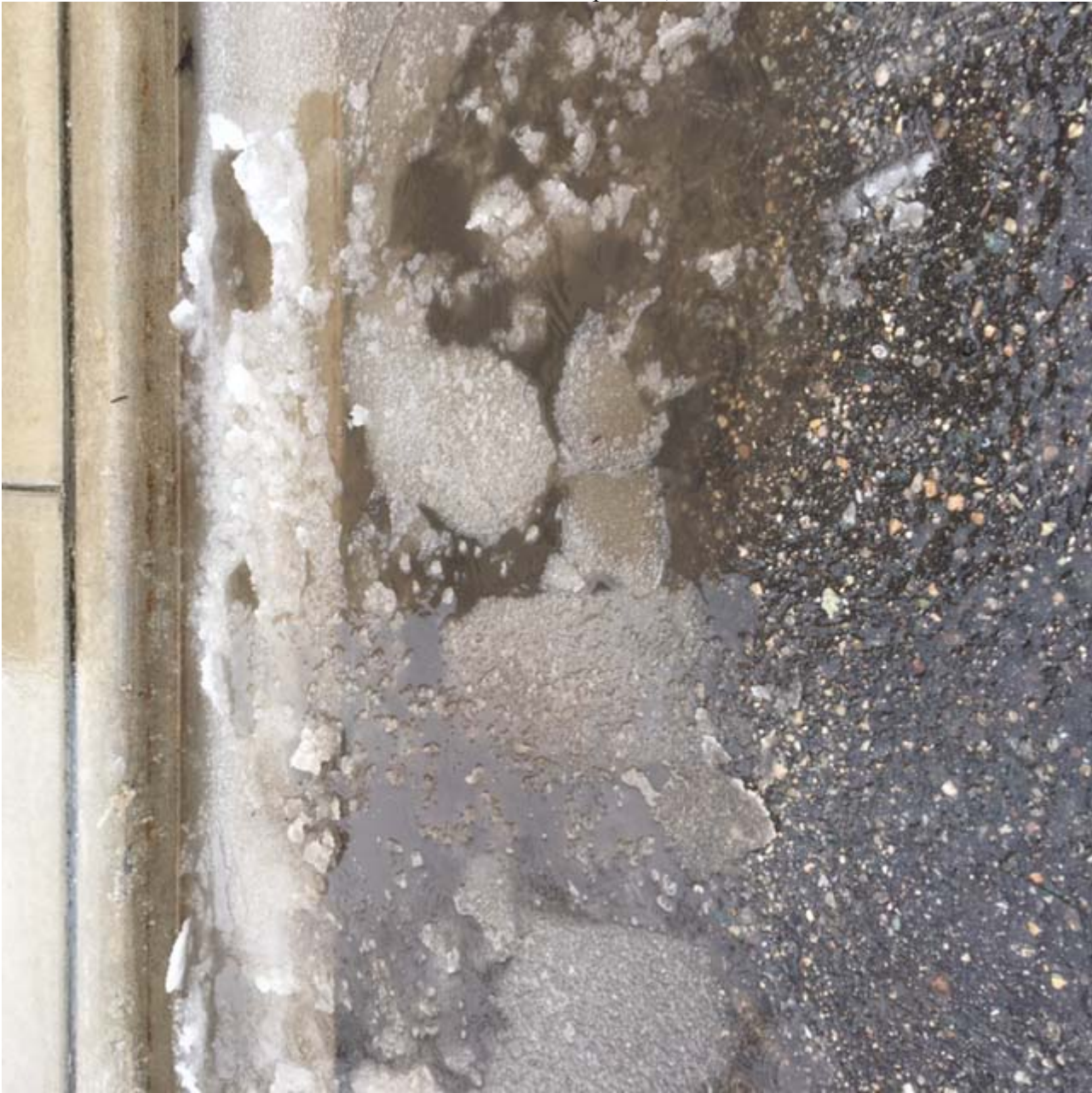
Pothole filled with snow and ice. Taken on or about April 10, 2015.
