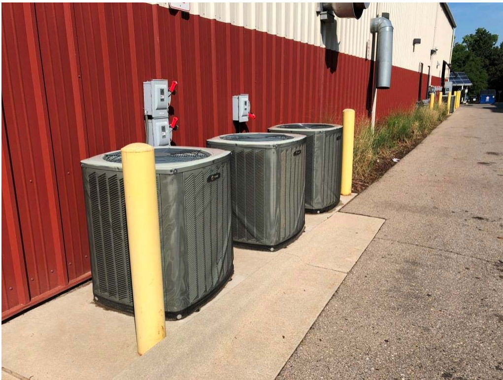
Exterior View – Mechanicals
