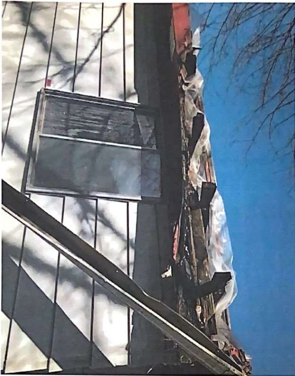
3601 DEERFIELD AVENUE PHOTOS SUBMITTED BY JERRY DUNHAM, CHIEF BUILDING INSPECTOR 4.25.2022
