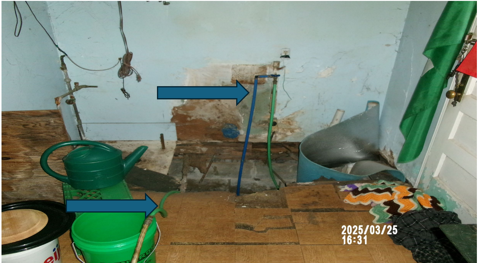
Garden hose used for plumbing
