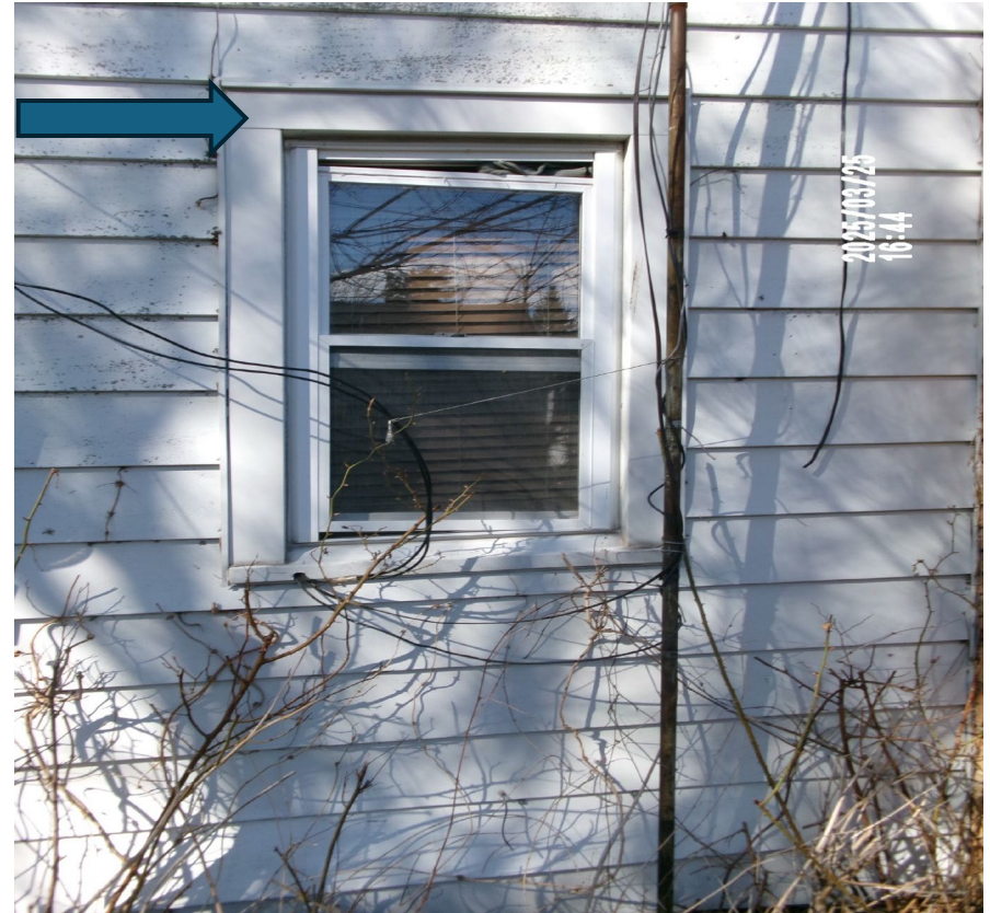
(right) Window level, however wall is not
