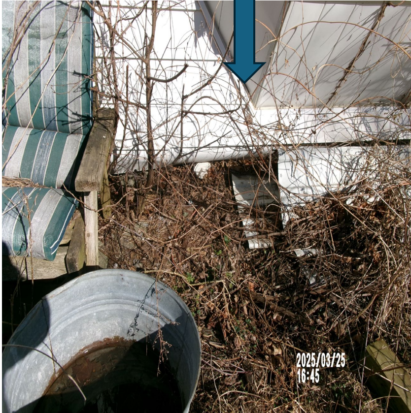
(above) rear wall separating from house.
