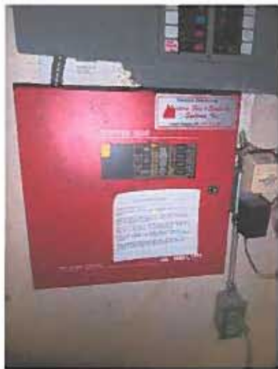
Example of an older fire alarm control panel (approximately 21 years old).
