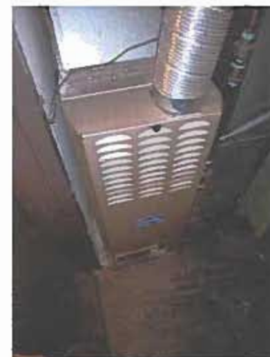
Example of a Carrier, gas-fired furnace serving common hallways/stairwells (one of five; similar furnace serving the leasing office).
