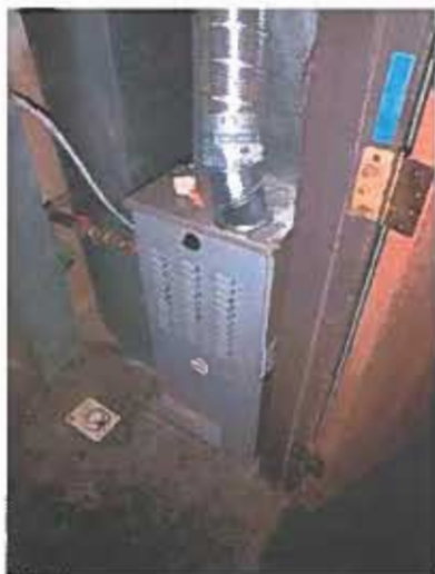
Example of an older Payne gas-fired furnace serving common hallway/stairwells (one of three).
