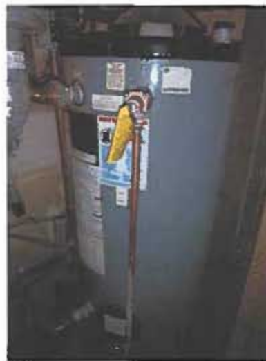
Example of an older (estimated 21 years old) RUUD, gas-fire domestic hot water tanks with a rated 199 MBH input capacity and 80-gallon storage tanks.
