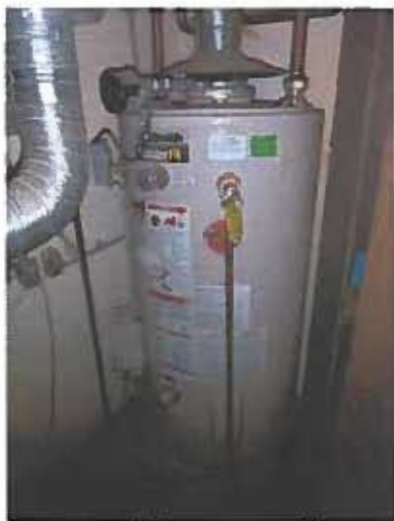
Example of an older (estimated 15 years old) A.O. Smith, gas-fire domestic hot water tanks with a rated 199 MBH input capacity and 80-gallon storage tanks.
