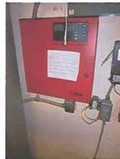
Example of an older fire alarm control panel (approximately 15 years old).
