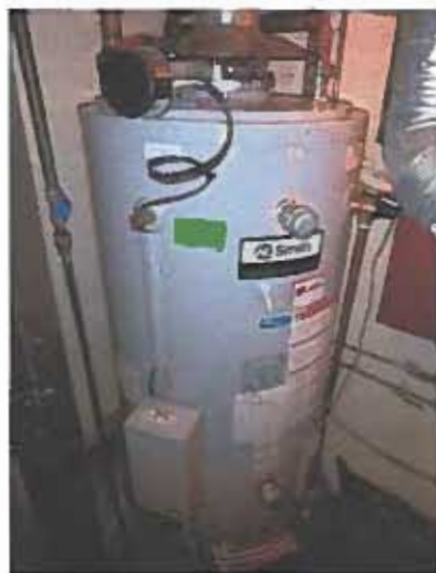
View of the newer A.O. Smith domestic hot water heater serving #611.
