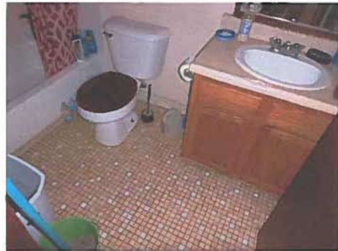
Typical bathroom fixtures and finishes.
