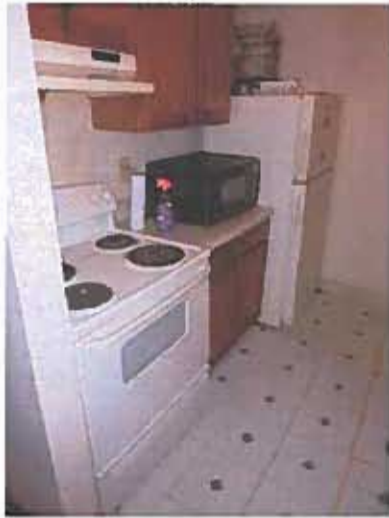
Typical dwelling unit kitchen cabinetry and appliances.
