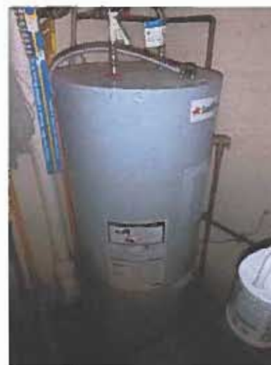
The electric tank serving the leasing office.
