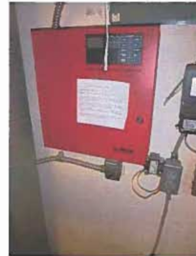
Example of an older fire alarm control panel (approximately 15 years old).
