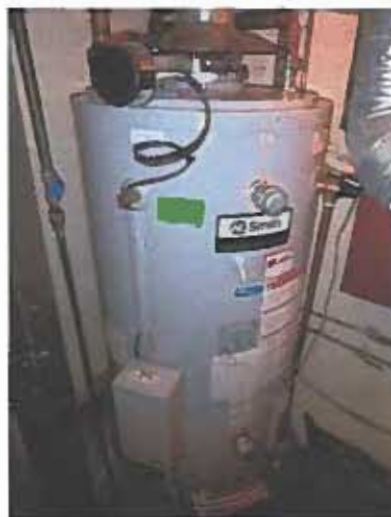
View of the newer A.O. Smith domestic hot water heater serving #611.
