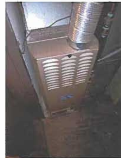
Example of a Carrier, gas-fired furnace serving common hallways/stairwells (one of five; similar furnace serving the leasing office).
