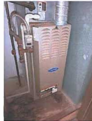
Typical unit level gas-fired warm air furnace located in a mechanical closet on the balcony/patio.
