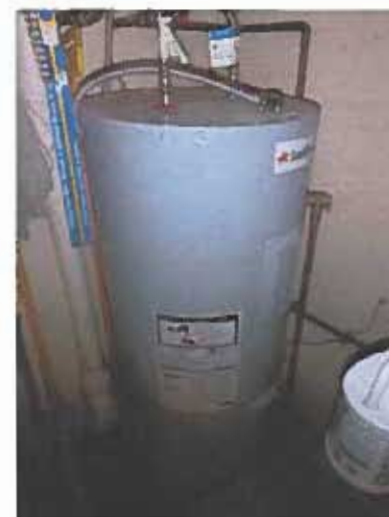
The electric tank serving the leasing office.
