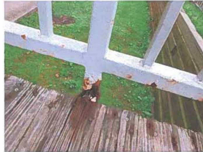
Close up of wood decking deterioration and rust damage to the railing system at a pedestrian bridge.
