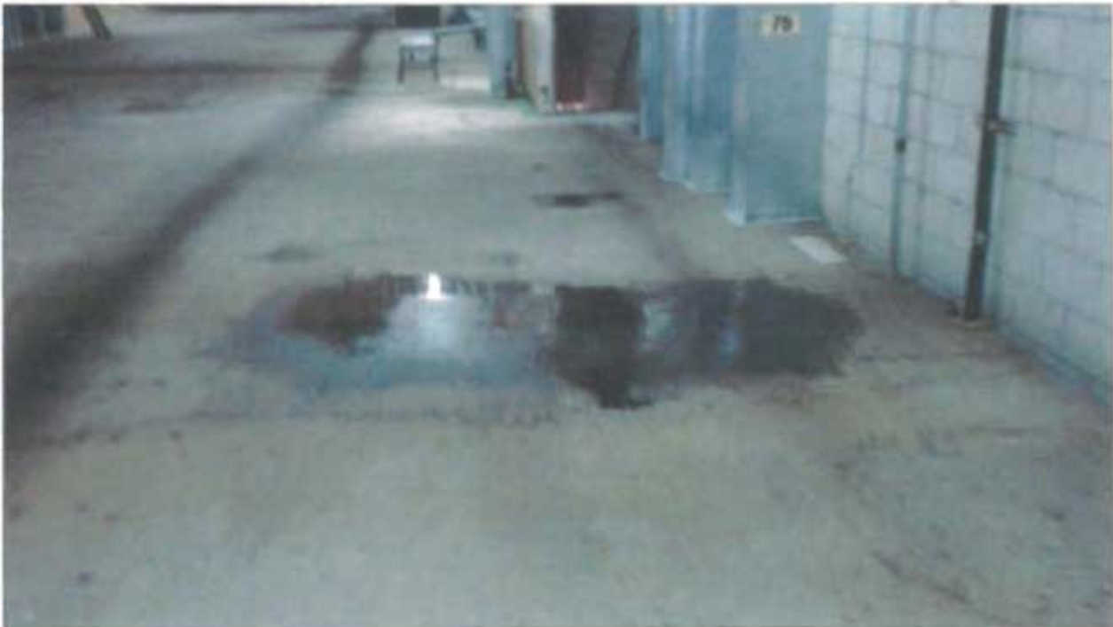
Roof Leaks at Rear Wall
