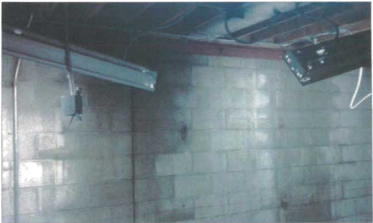
Roof Leaks at Rear Wall
