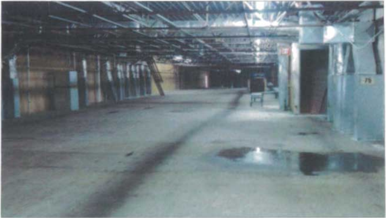
Mezz Level Roof Leaks
