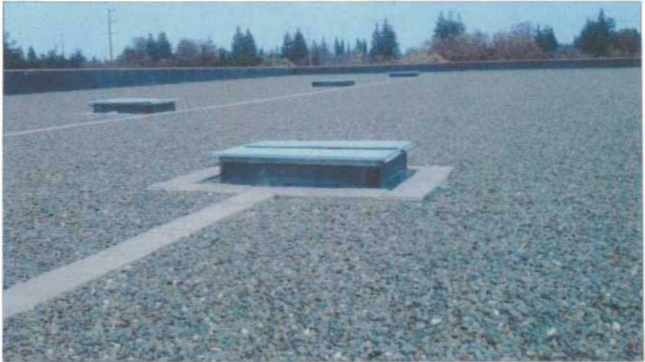
Roof with missing HVAC Units
