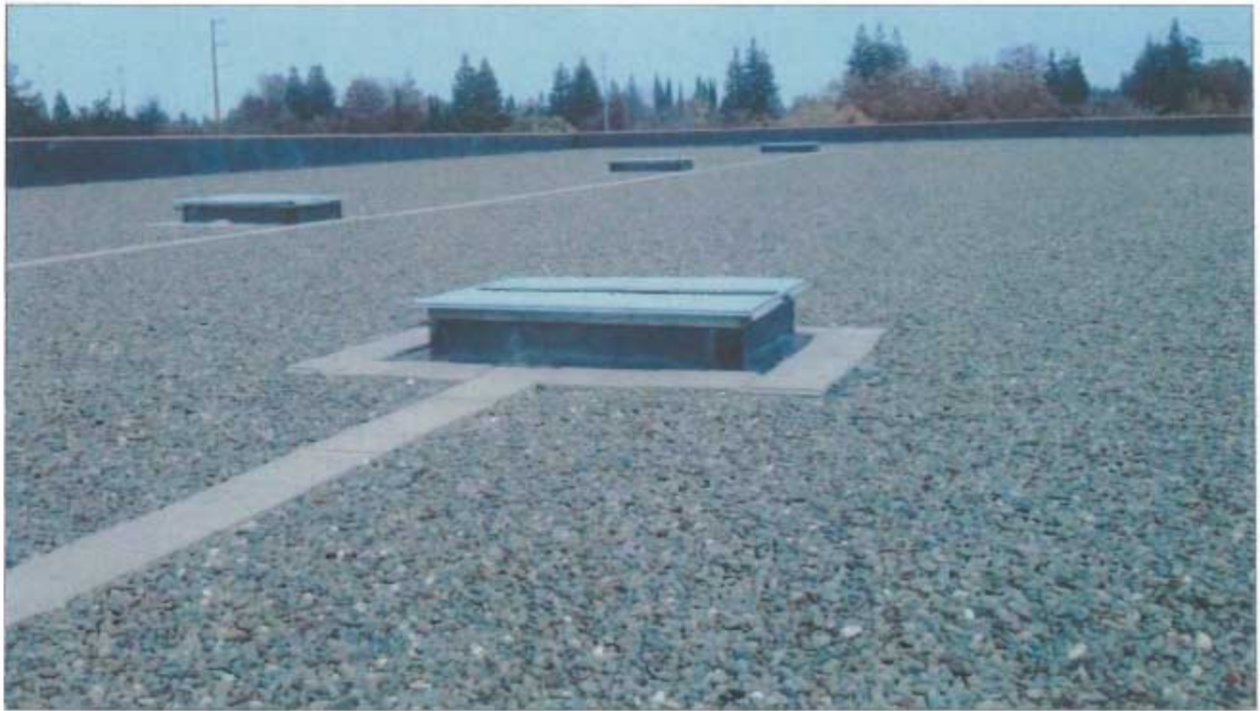
Roof with missing HVAC Units
