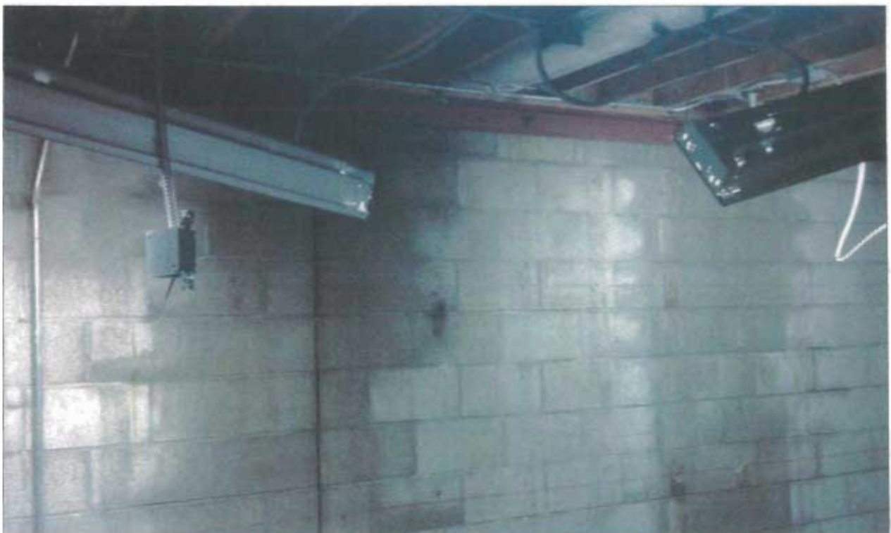
Roof Leaks at Rear Wall
