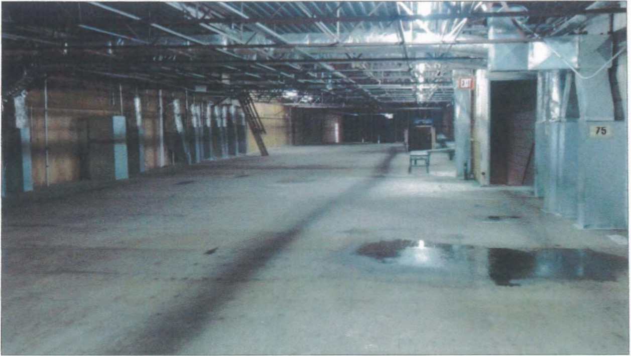
Mezz Level Roof Leaks
