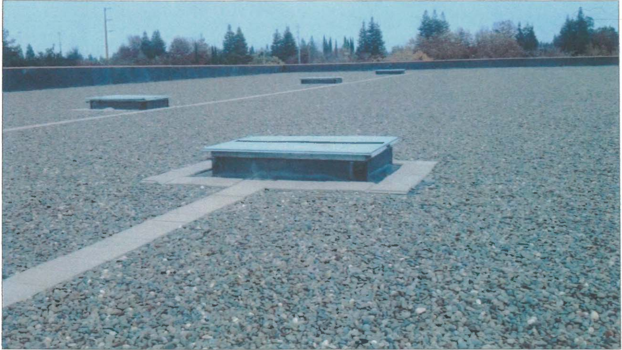
Roof with missing HVAC Units
