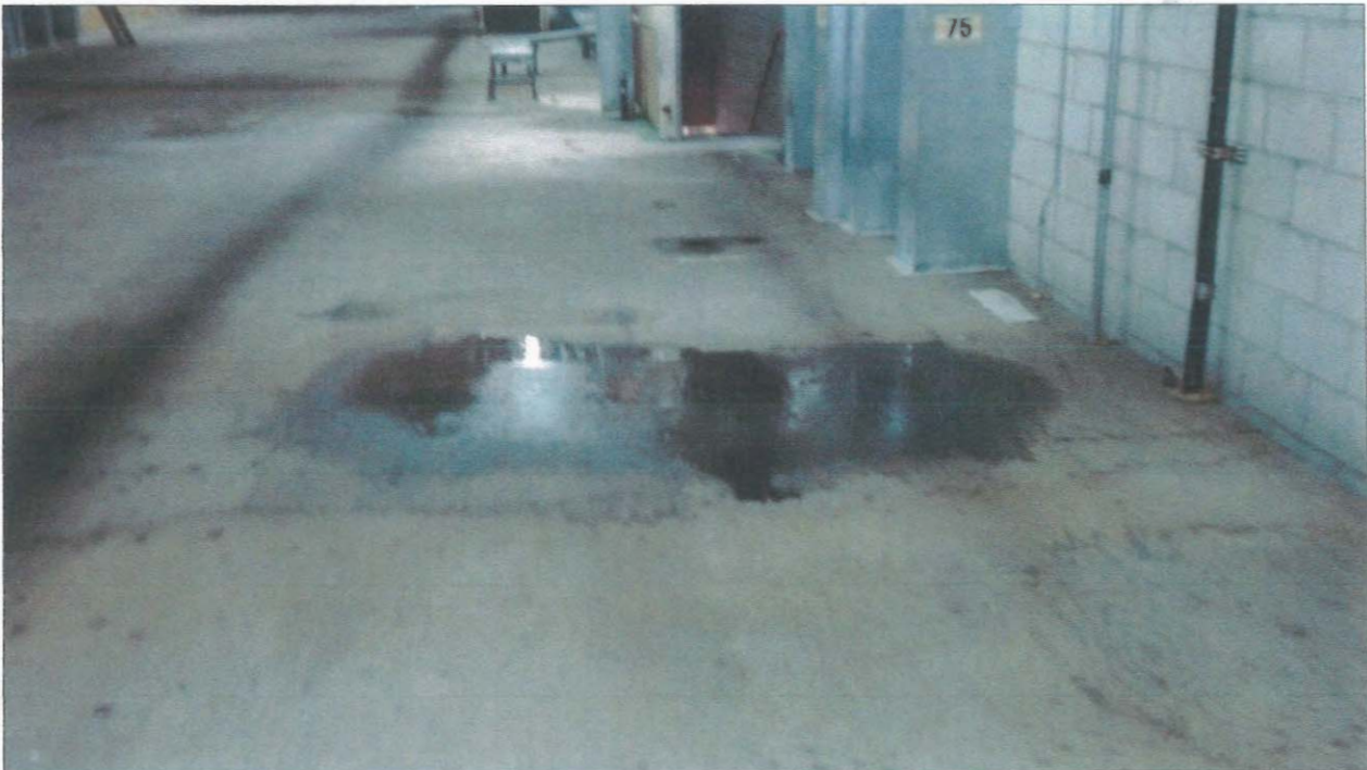
Roof Leaks at Rear Wall
