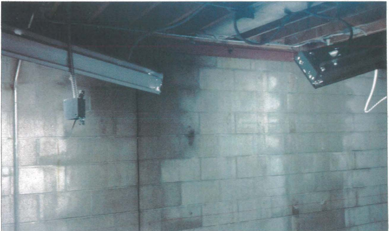
Roof Leaks at Rear Wall
