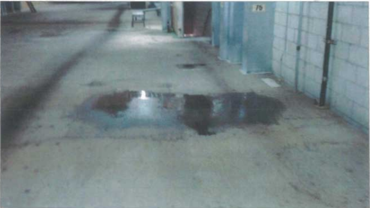
Roof Leaks at Rear Wall
