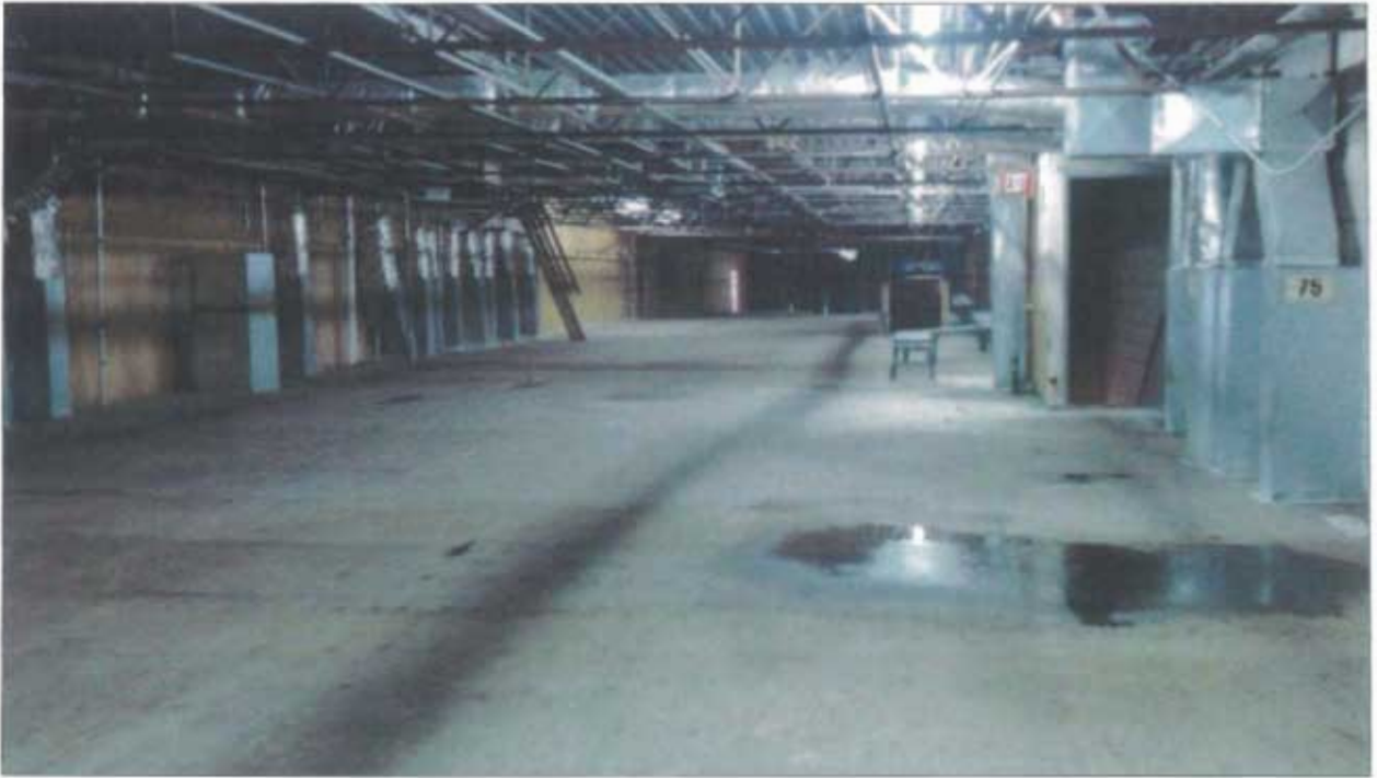
Mezz Level Roof Leaks
