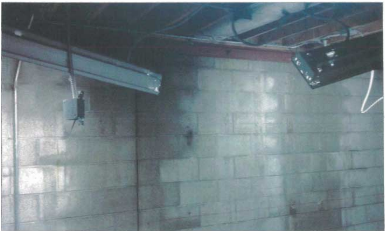
Roof Leaks at Rear Wall
