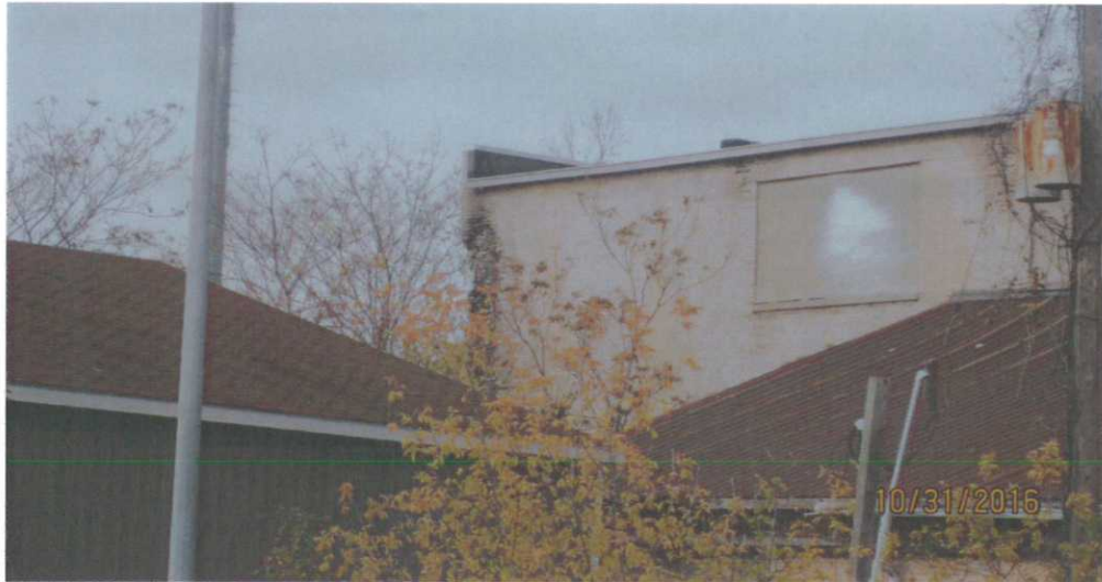
PHOTO: 5 DATE: 10/31/2016 SUBJECT: Eroded brick on the southwest corner of building.
