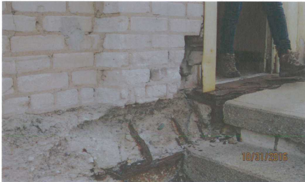
PHOTO: 3 DATE: 10/31/2016 SUBJECT: Eroded foundation on west side of building.
