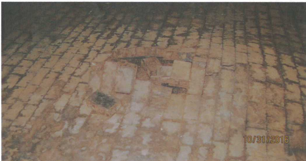
PHOTO: 10 DATE: 10/31/2016 SUBJECT: Buckled wood flooring located in the basement of the building.
