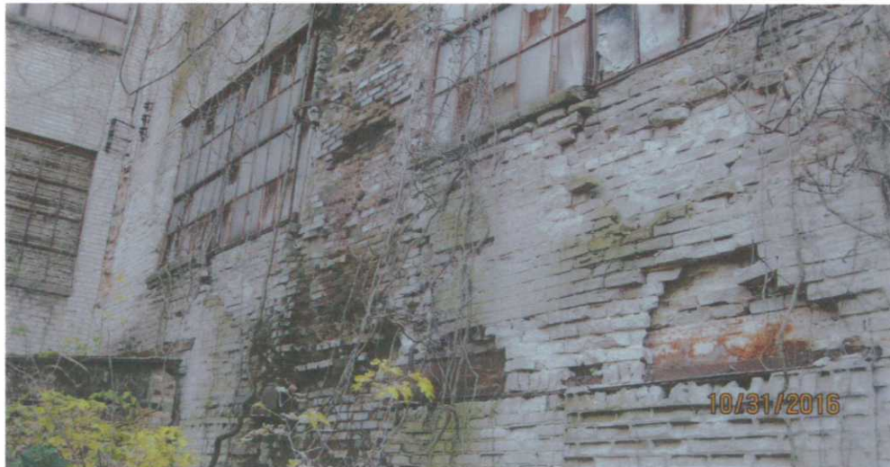
PHOTO: 4 DATE: 10/31/2016 SUBJECT: Eroded brick on the southwest side of building.
