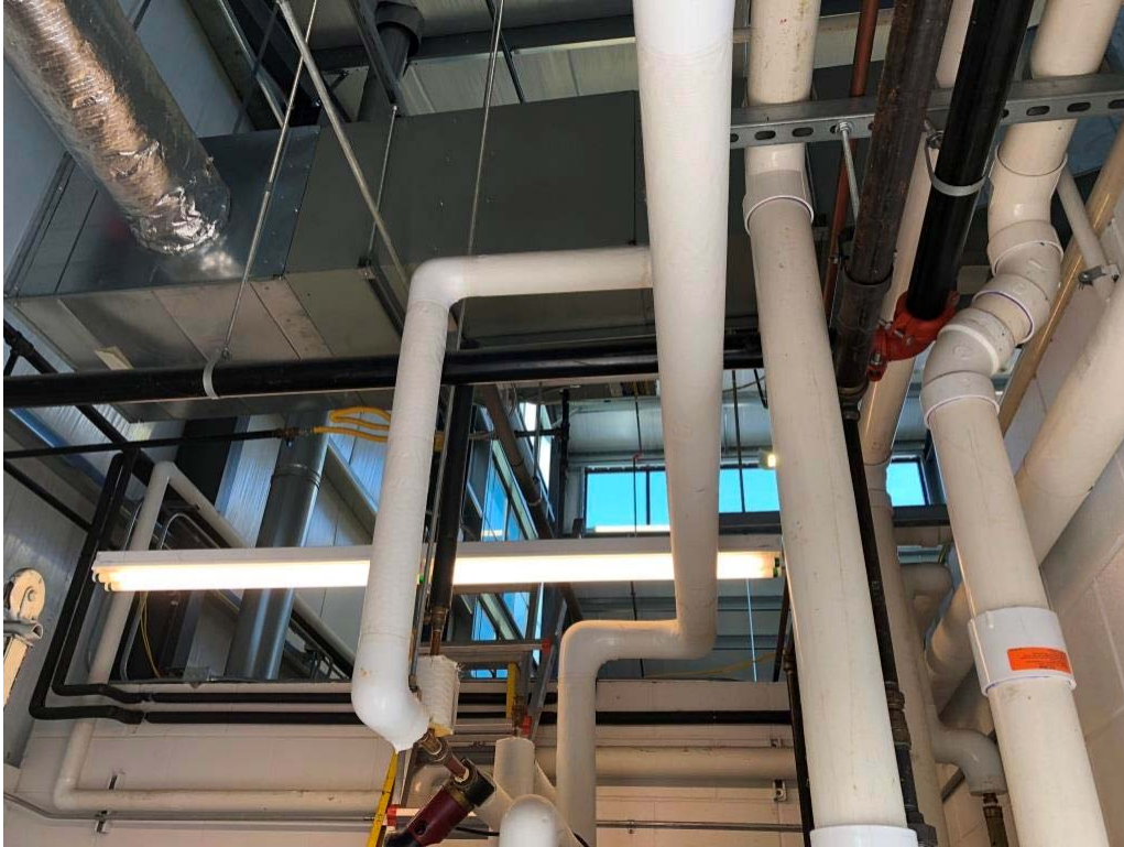
Interior View – Mechanicals
