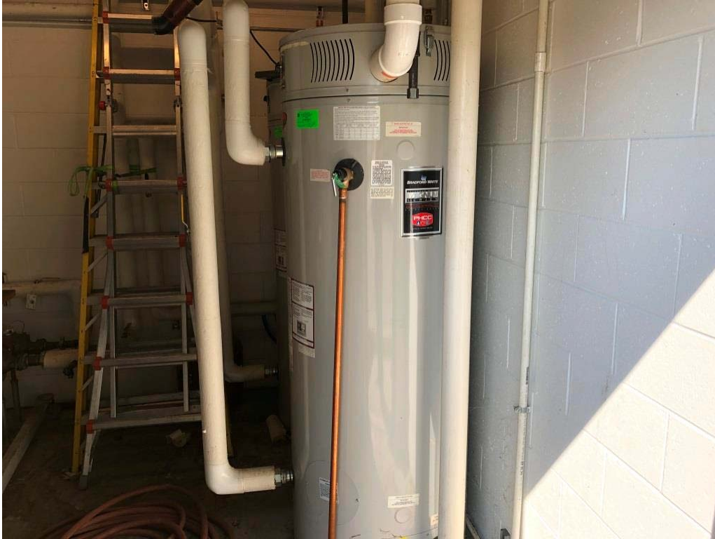
Interior View – Mechanicals
