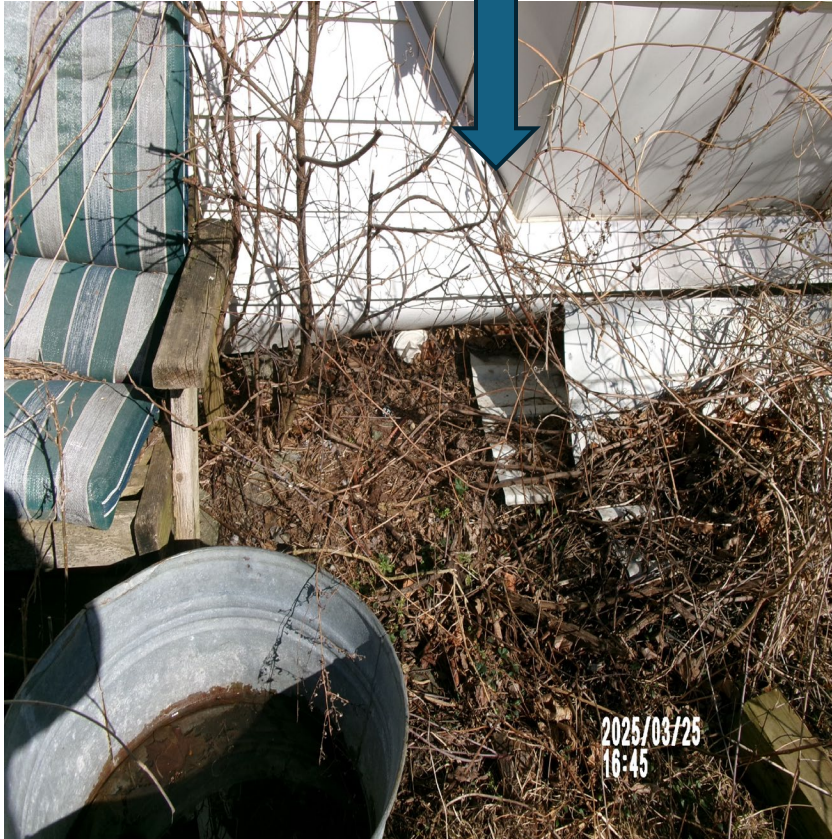
(above) rear wall separating from house.
