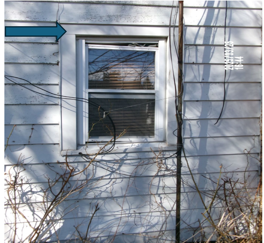
(right) Window level, however wall is not
