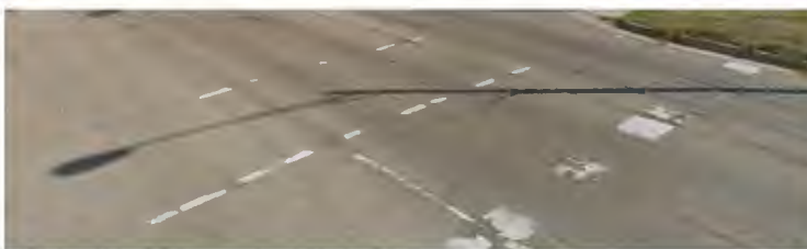
Figure 16: Significantly Worn Stop Bar and Crosswalk
