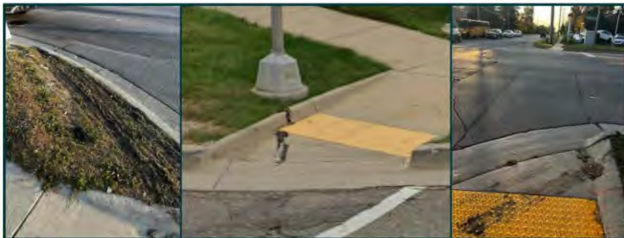
Figure 15 - Tire tracks outside the roadway at Aurelius Road (left), broken curb ramps at Dunckel Road (Center), and tire tracks outside the roadway at Pennsylvania Avenue (right)
