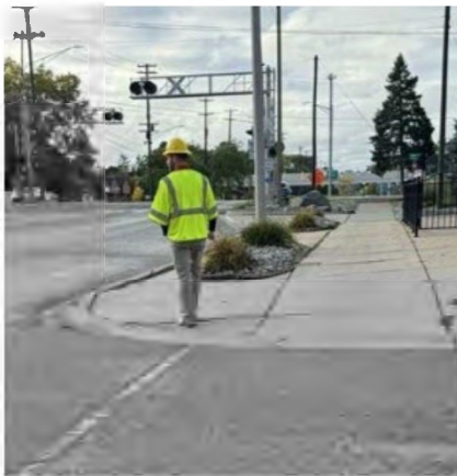
Figure 12: Missing ADA Tactile Warning Surface
