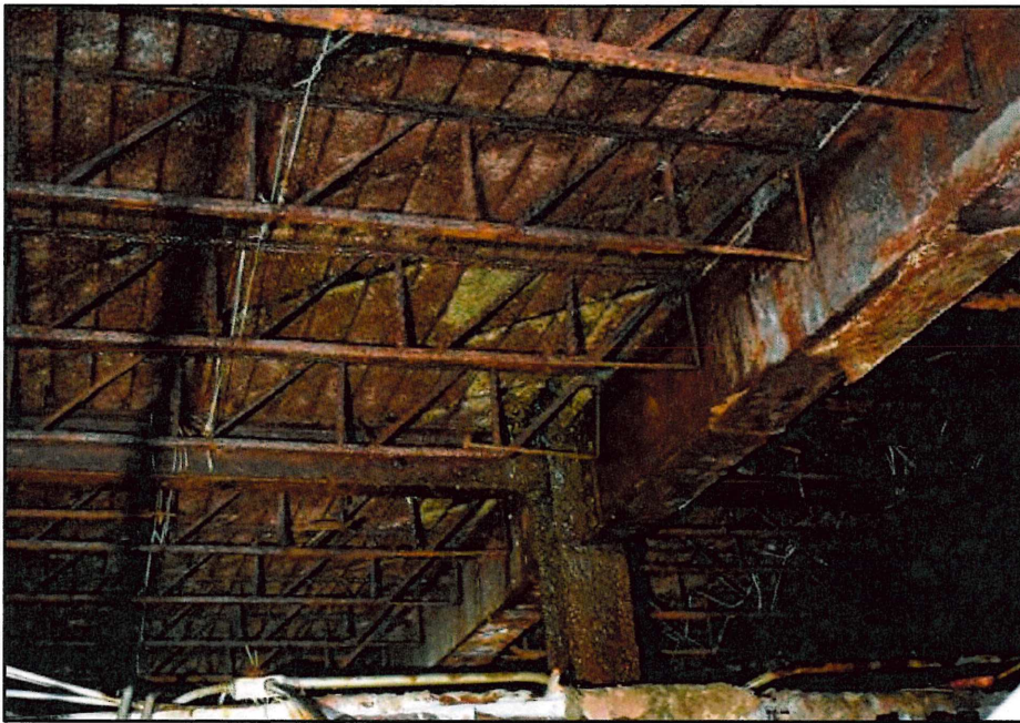
PHOTO NO. 5: Supported floor framing with surface corrosion and pack-rust formation.
