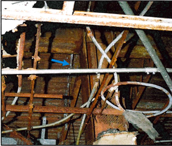
PHOTO NO. 6: Active leak (blue arrow) near beam-column framing.
