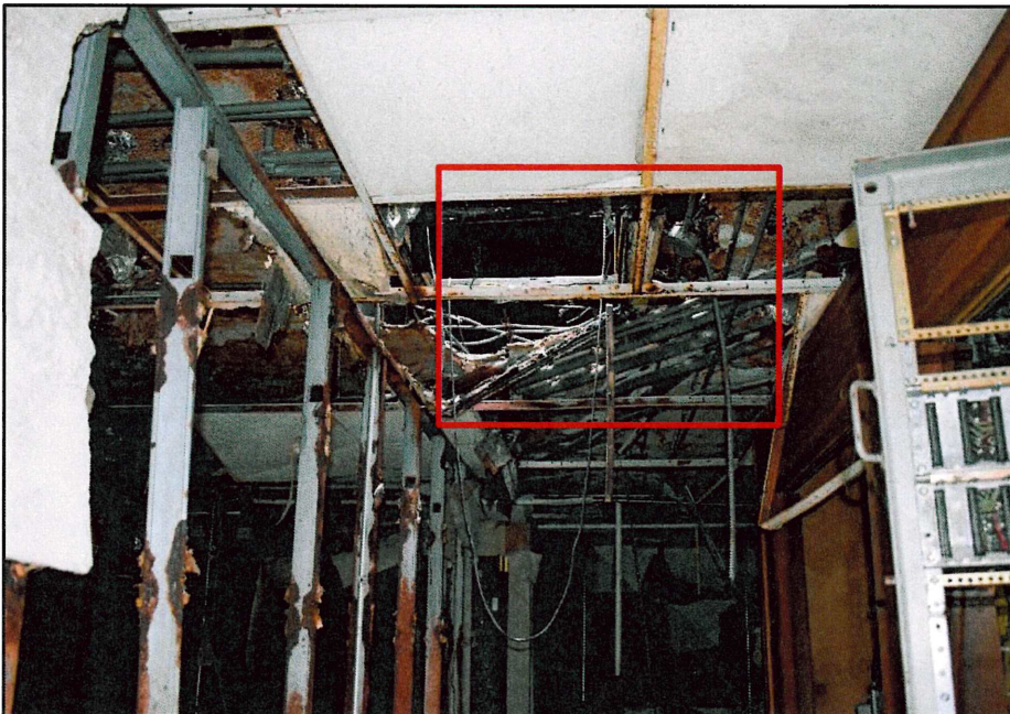
PHOTO NO. 9: Representative hole in roof (daylight shining through indicated by red rectangle).
