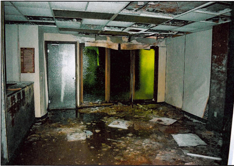
PHOTO NO. 7: Ponding water on second-floor.
