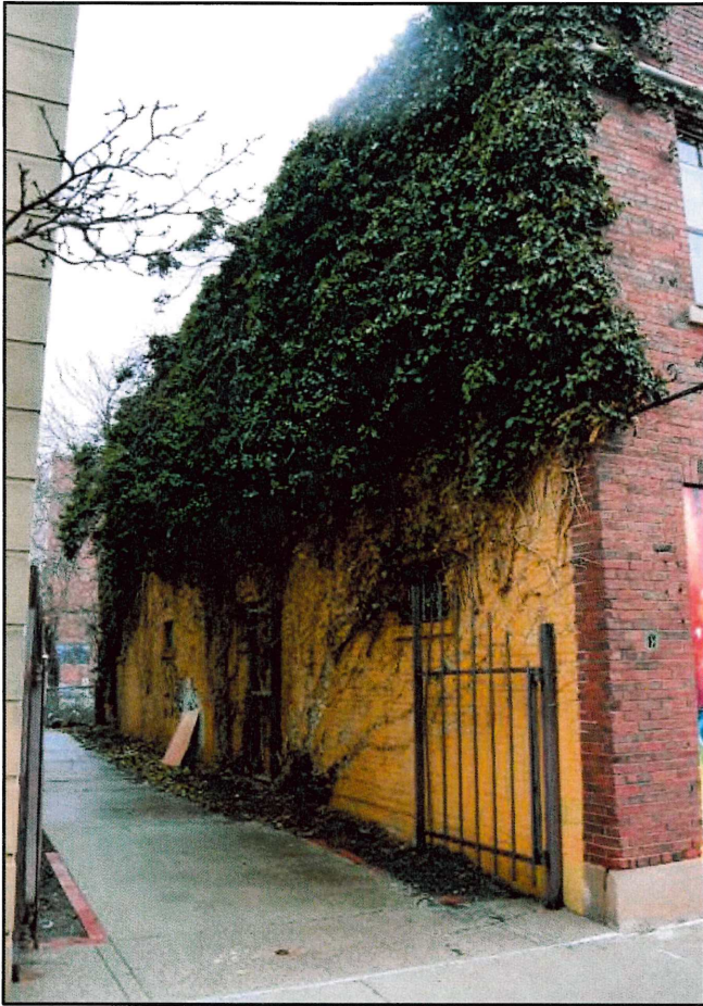
PHOTO NO. 12: Ivy growth partially concealed west wall south half.
